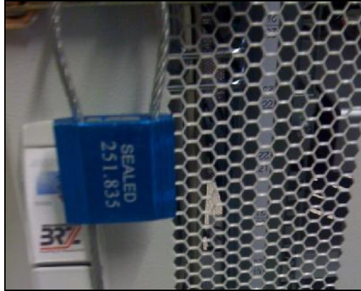
Figure 4: Sealed security rack
